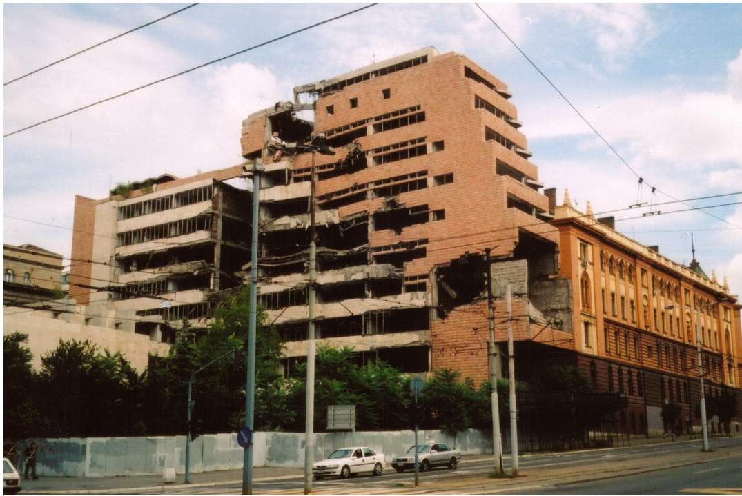
Remains of the Yugoslav Army headquarters bombed by NATO during the aerial campaign in 1999
